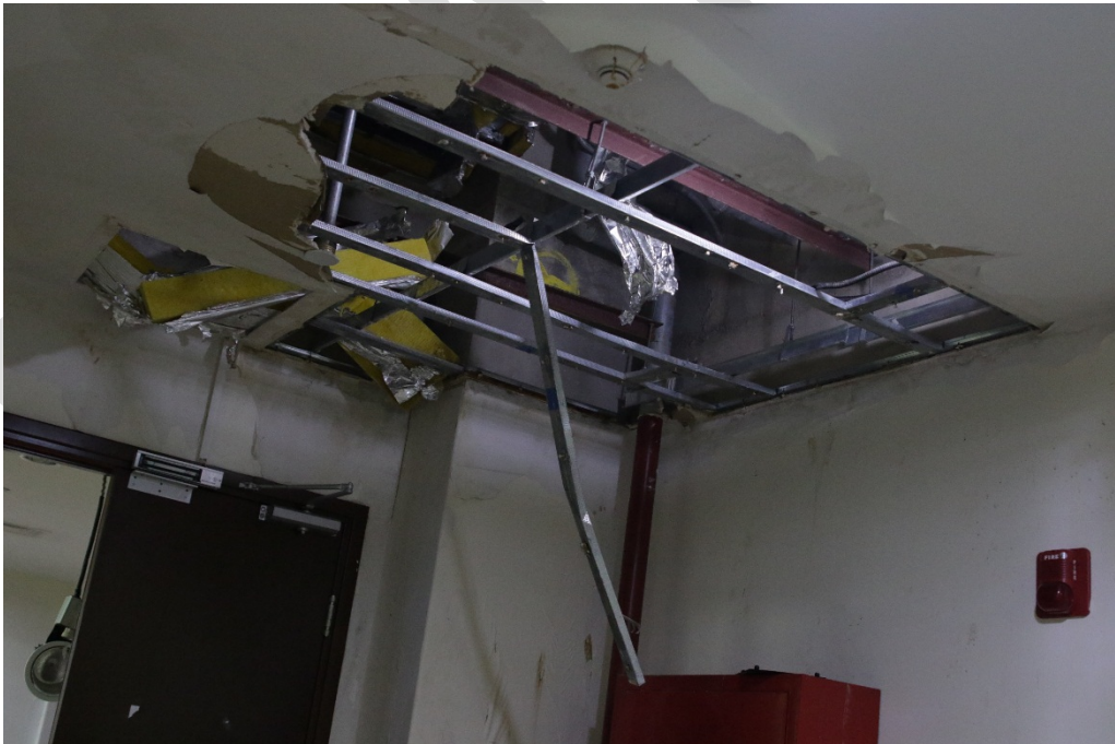
FIGURE 23 DAMAGED CEILING AT VELODROME
