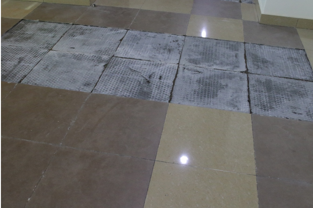
FIGURE 21 DAMAGED TILES AT THE VELODROME (LOWER LEVEL)
