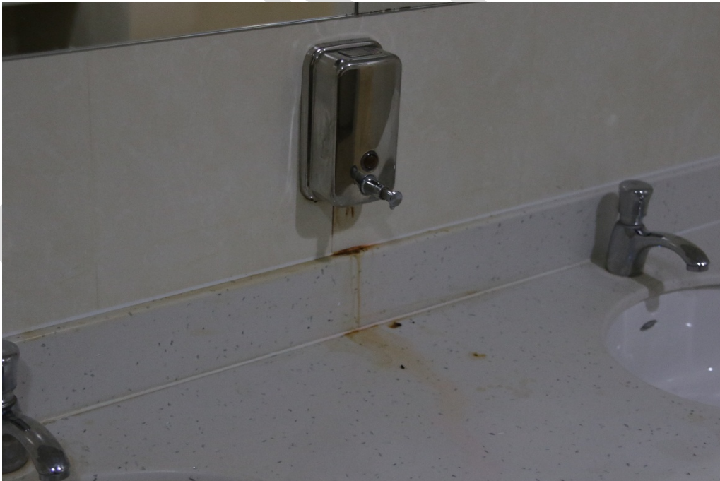
FIGURE 23 RUST DAMAGE IN BATHROOM AT VELODROME
