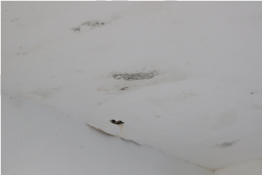
FIGURE 14 WATER DAMAGE ON CEILING AT NATIONAL AQUATIC CENTRE
