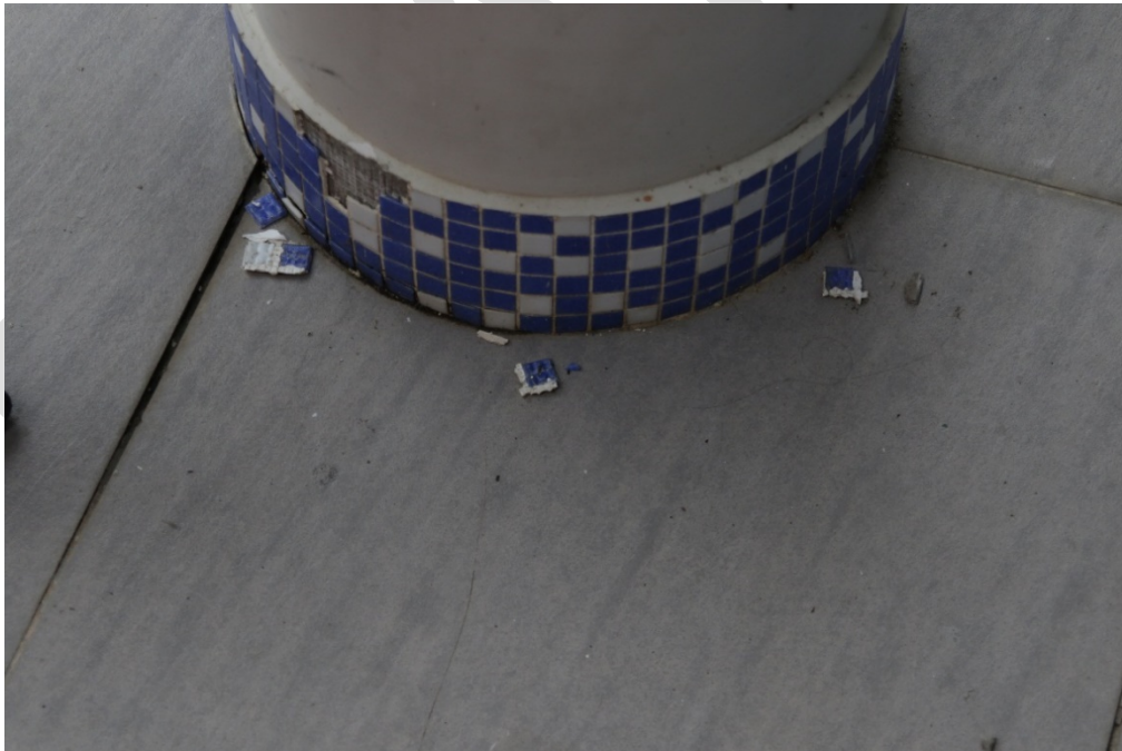
FIGURE 10 TILES FALLING OFF COLUMN AT NATIONAL AQUATIC CENTRE
