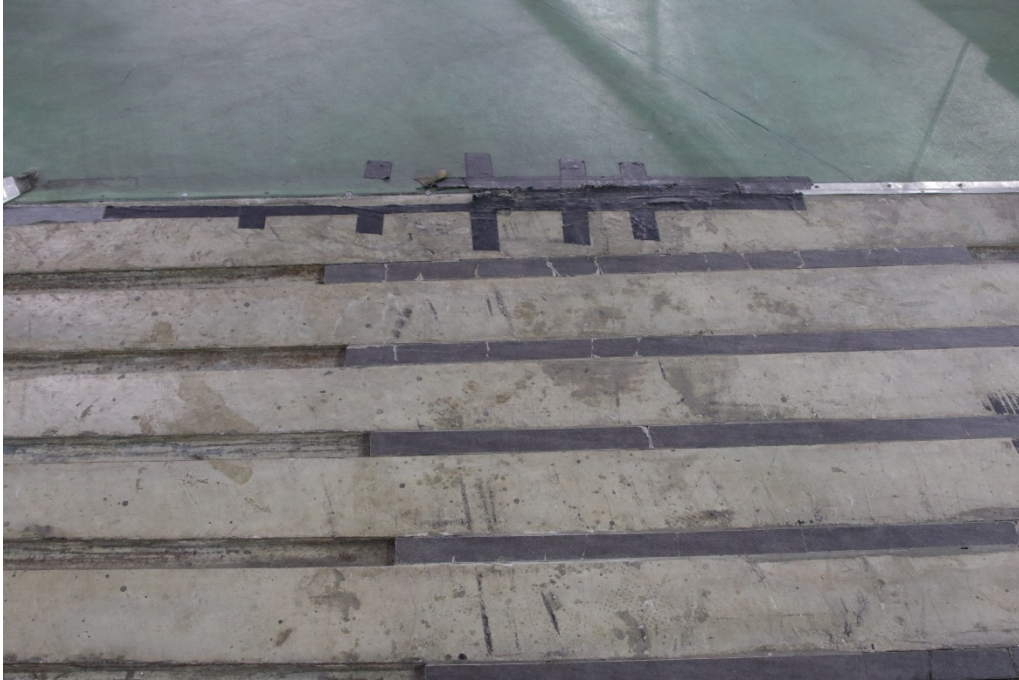
FIGURE 15 DAMAGED FLOORING AT VELODROME
