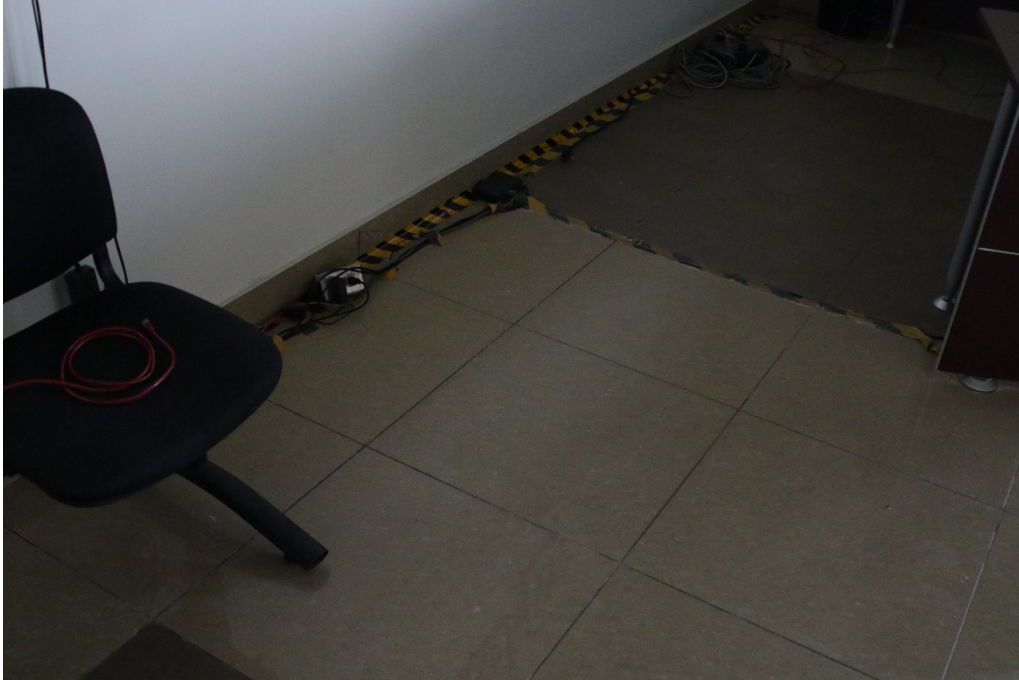
FIGURE 24 DAMAGED TILES AT VELODROME
