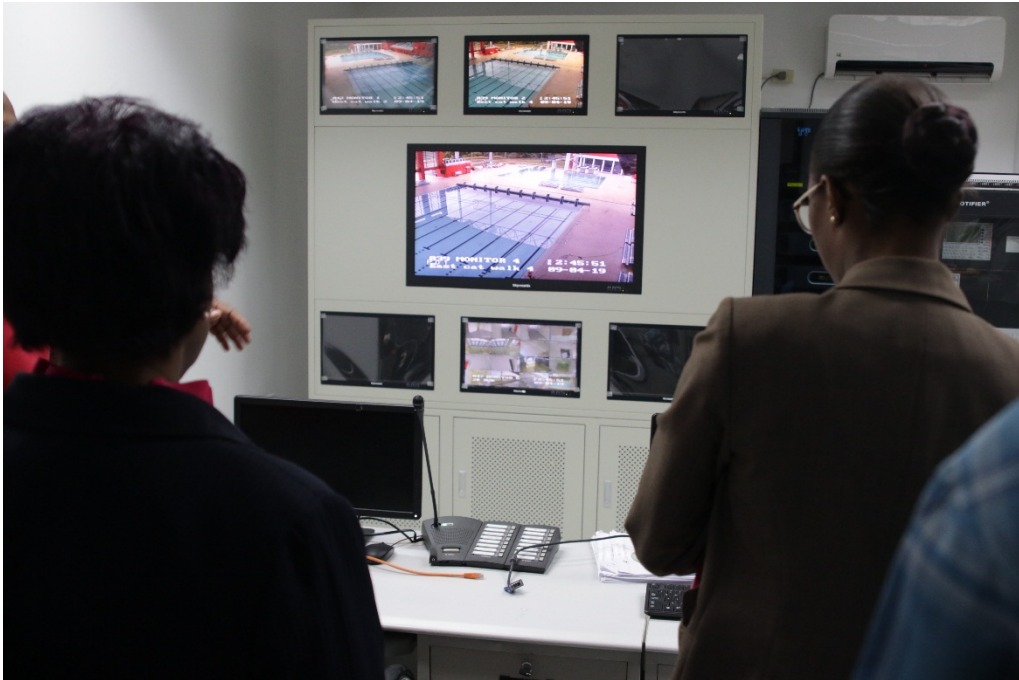
FIGURE 7 CONTROL ROOM SCREENS
