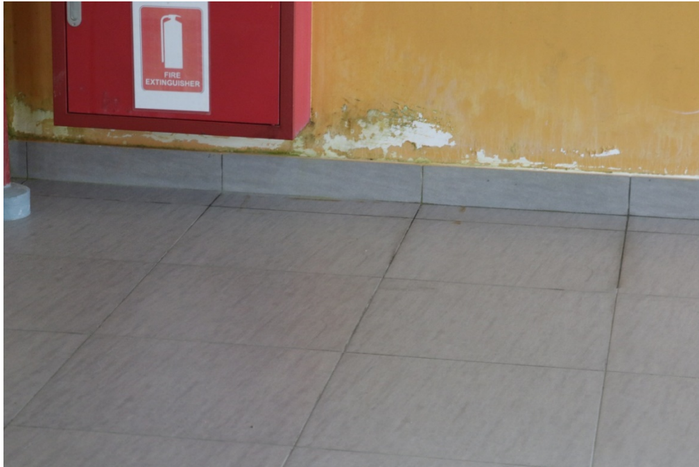
FIGURE 11 WATER DAMAGE AT NATIONAL AQUATIC CENTRE
