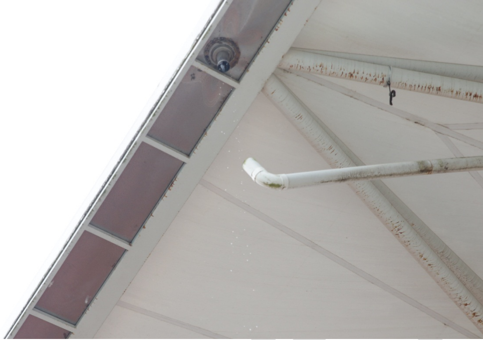
FIGURE 5 LEAK OVER BLEACHERS AT NATIONAL AQUATIC CENTRE
