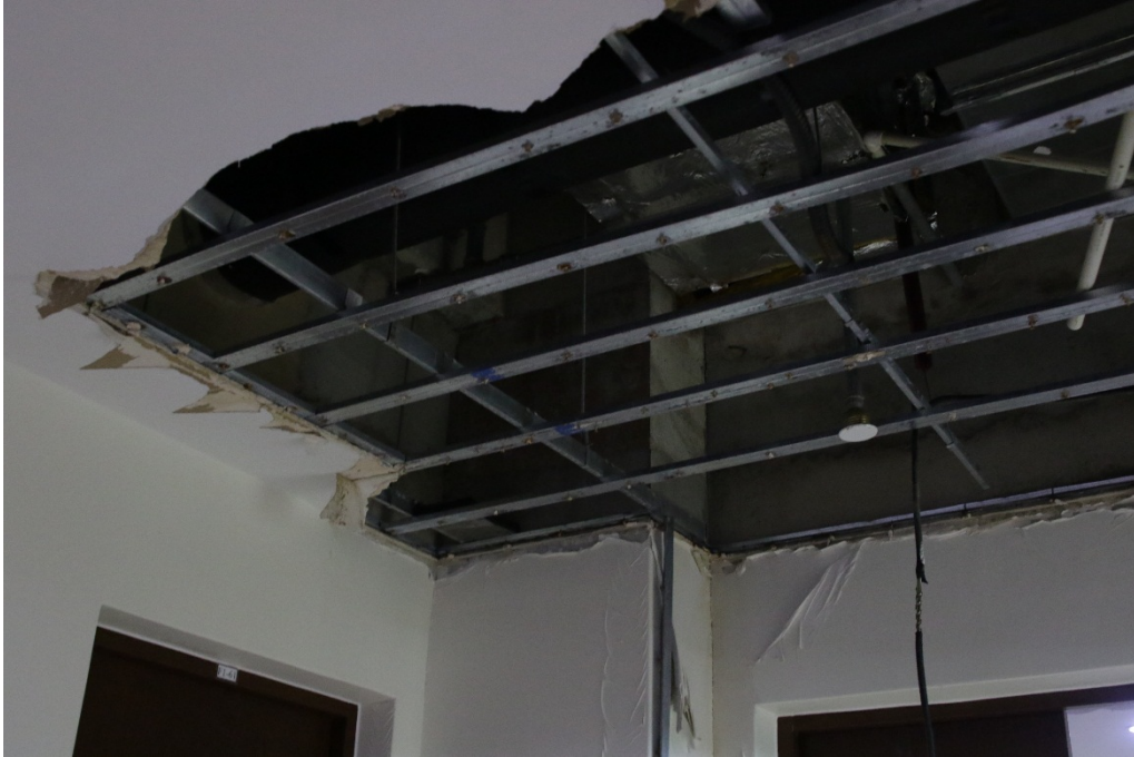
FIGURE 22 DAMAGED CEILING AT VELODROME
