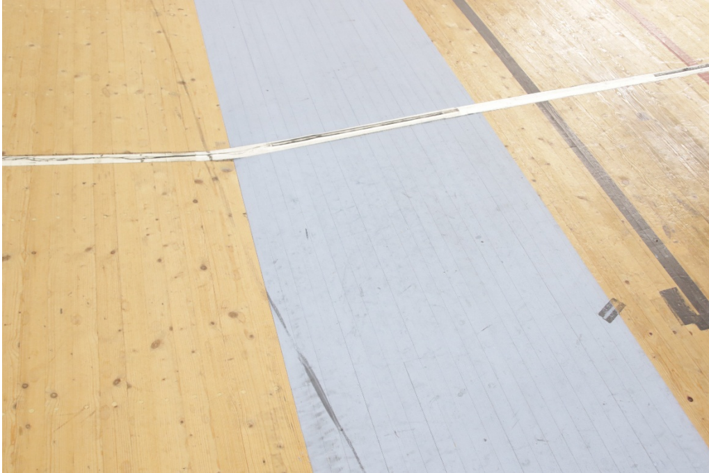
FIGURE 17 DAMAGED FLOORING AT VELODROME
