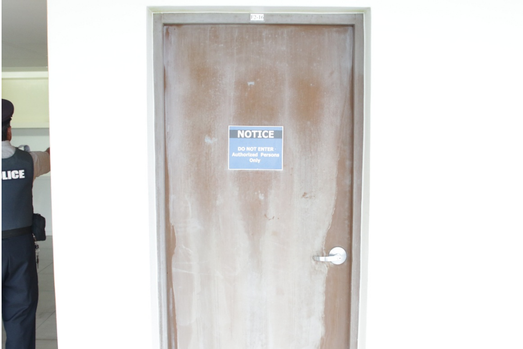
FIGURE 13 CONDENSATION APPEARING ON DOOR AT NATIONAL AQUATIC CENTRE
