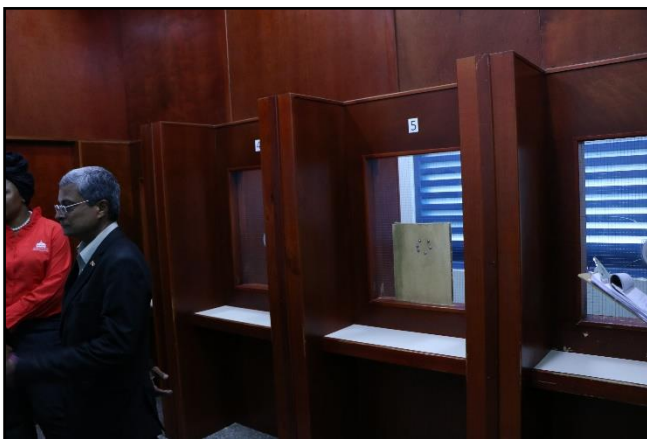
Figure 34: Cubicles with broken speaking areas at the Visitors Area
